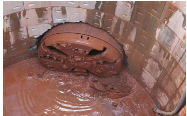
Tunnel Boring Machine (TBM) emerges into Powderham reception shaft after its 2km drive under the River Exe estuary to create a gas pipeline tunnel. (photo - D Laming)
