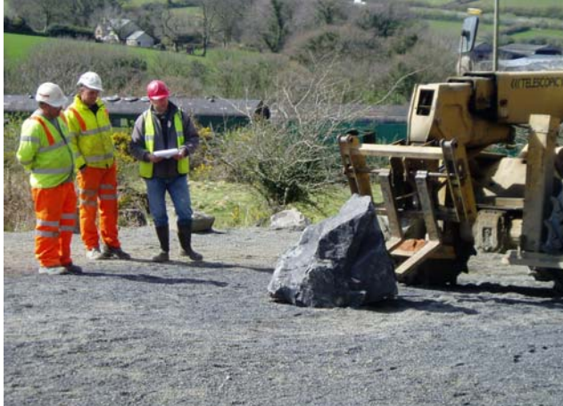
Placing the first boulder - Phil Stephenson supervises the selection of boulders from the quarry and the arrangement of the Rock Park area, with assistance from Bardon Aggregates and Bardon Contracting.
